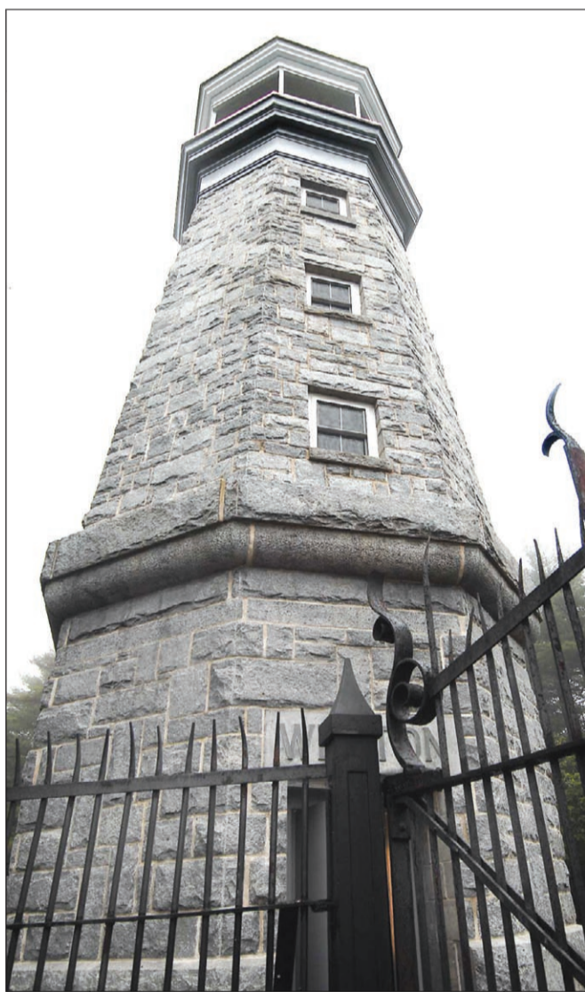
The interior and exterior masonry have been re-pointed as well as new windows and painting as part of the restoration on the Weston Observatory in Manchester.
